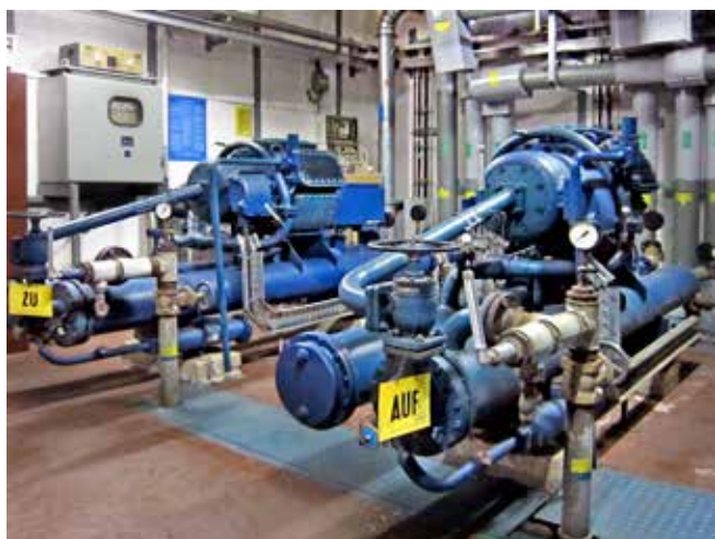
Compressors for the compressed-air tanks. Photo Tim Wellburn
